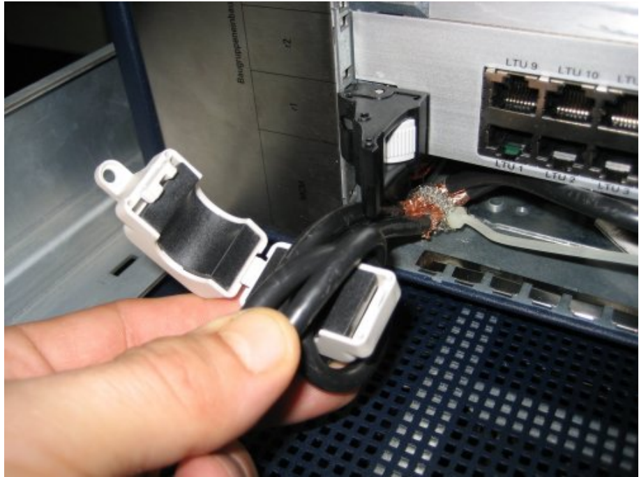
Figure 46: Looping the DC cables through the ferrite core
