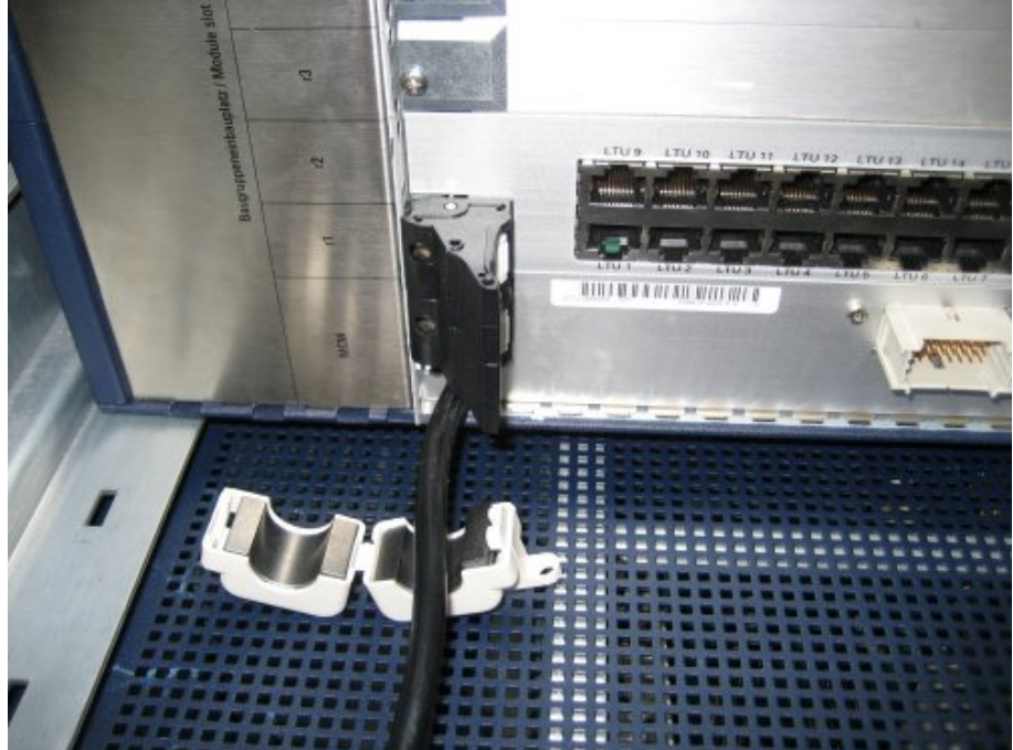
Figure 39: Opened ferrite core below AC cable
