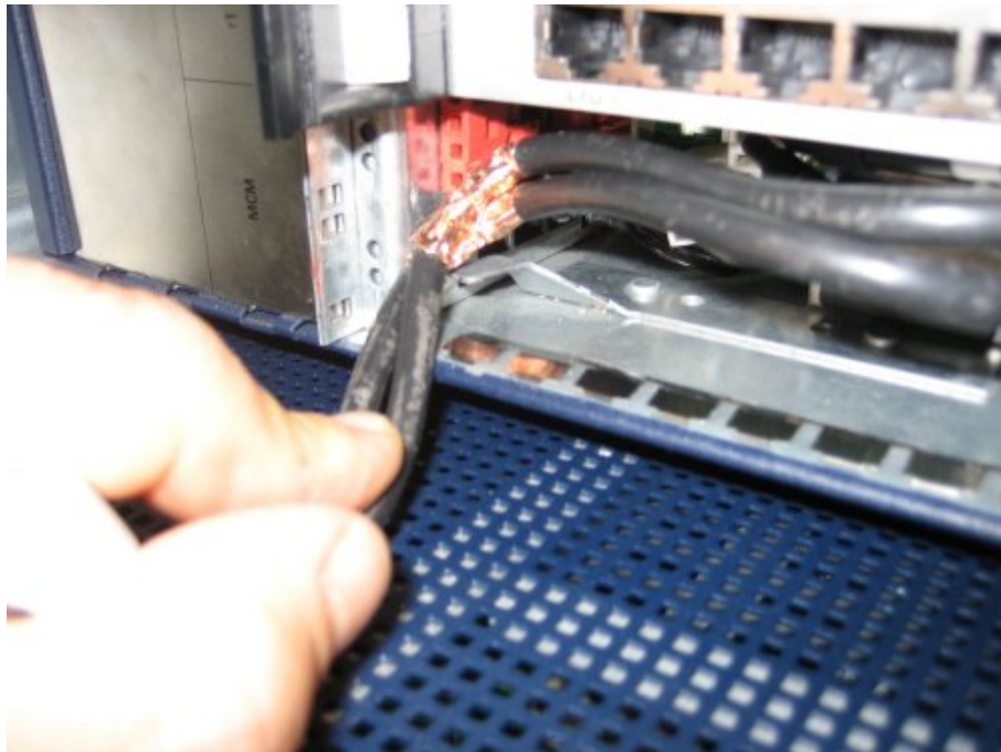
Figure 42: Stripped DC cable
